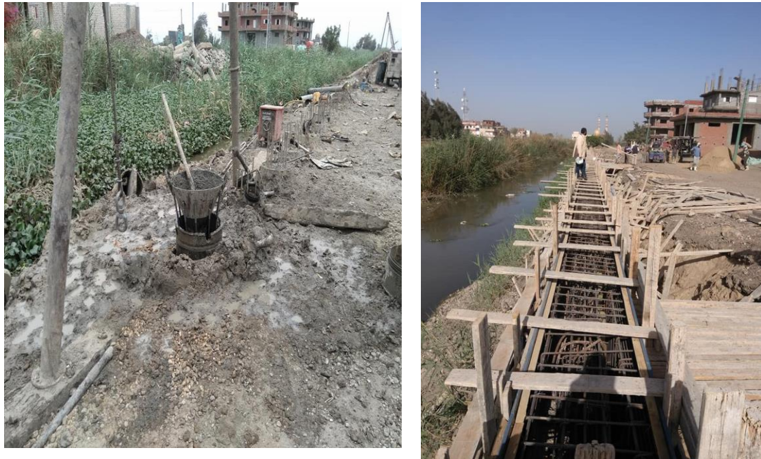
Figure 23: stages 1,2 of method C protection of slope failure the Abu Homs drain
