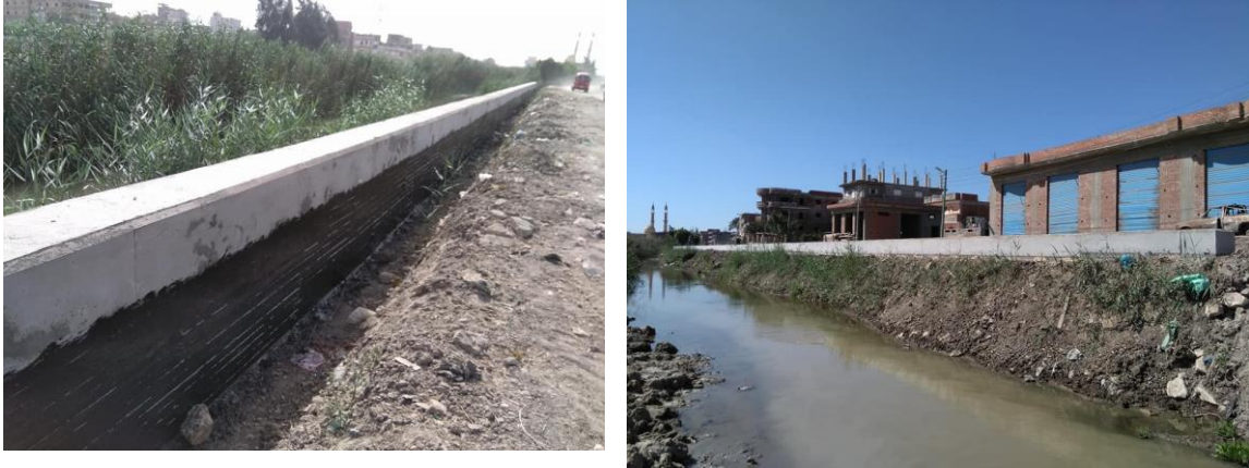
Figure 24 stages 3,4of method C protection of slope failure the Abu Homs drain
