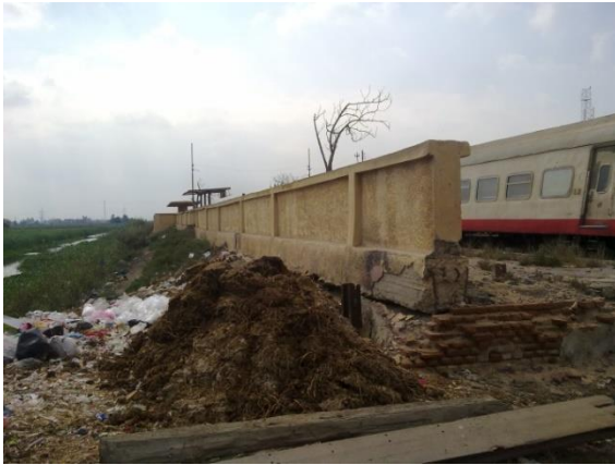
Figure 2 : Abu Hummus Drainage failure 01- Sahaly
