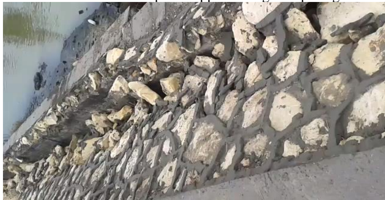
Figure 19: section(A-A) of Method (B) of Protection of slope failure the Abu Homs drain
