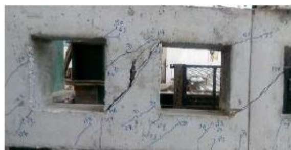
(c) Zone A of Beam B2
