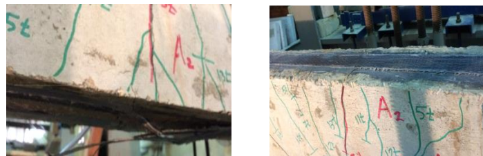
Fig. 9d: the mode of failure for Specimen A2
