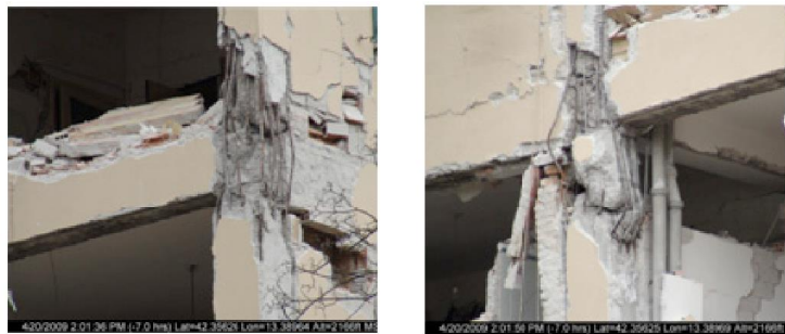
Fig. 2 Severe damage in beam column connection in RC building, L'Aquila Earthquake, Italy -2009. [3]
