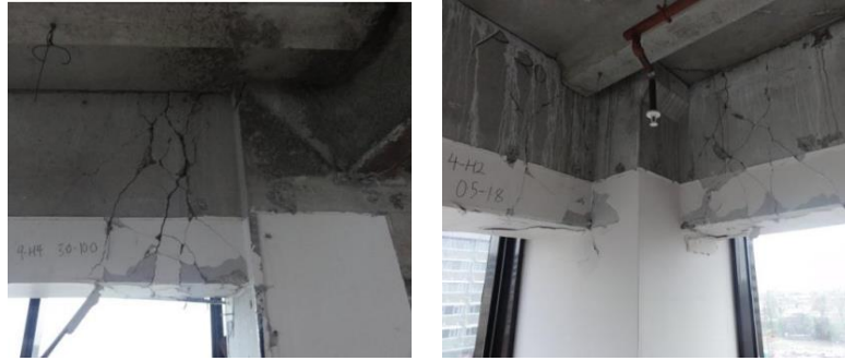
Fig. 4 Damage of ductile Beam Column Joint at the Price Waterhouse Coopers Building-New Zealand at 22 Feb 2011 Christchurch earthquake [6]
