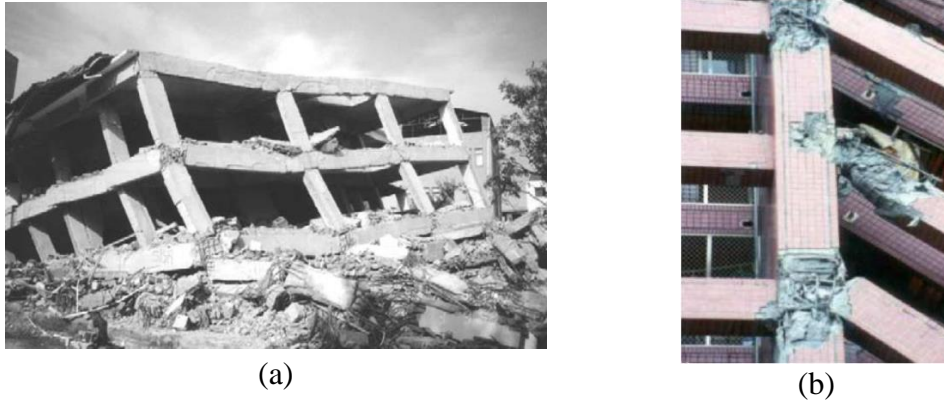
Fig. 1 (a) Collapsed building from the August 17, 1999 Kocaeli Earthquake [5] (b) Damage to 15-story building in the September 21, 1999 Chi-Chi Taiwan Eq.
