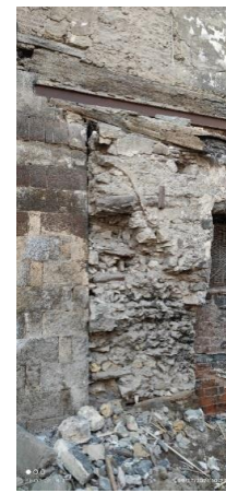
(c) Signs of deterioration and missing parts.
