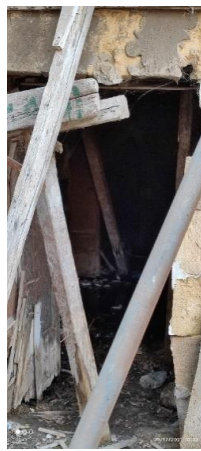
(b) Signs of dampening and high ground water table.
